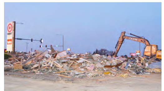
Demolition of the former Perkins building has begun at the Chick-fil-A site. Shorewood Development is also moving ground at the strip center to prepare for construction.
